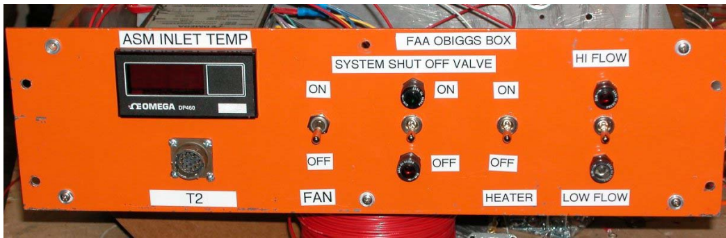
FIGURE 6. FRONT PANEL OF THE FAA OBIGGS CONTROL BOX
