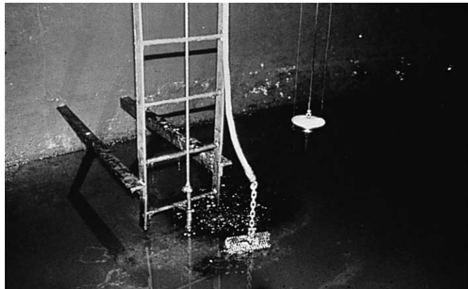
Figure 4a Example of sludge build-up at the bottom of a fuel storage tank.
